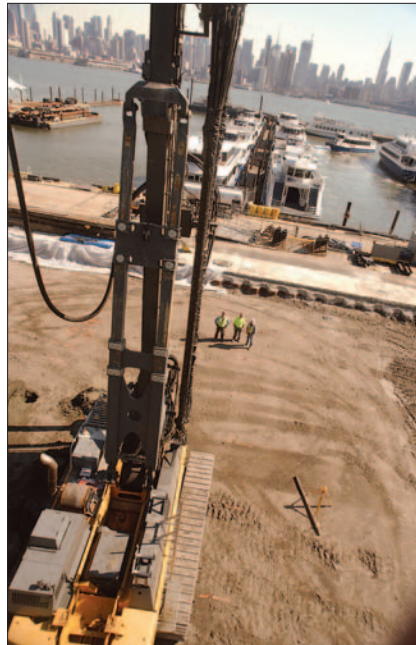
▲ Ground Improvement. Henley on Hudson residential development relies heavily on CMCs for foundation soil consolidation.
