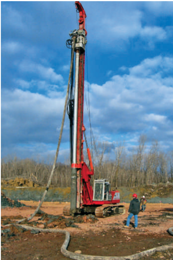
Menard installed Controlled Modulus Columns to improve the ground at a site with very soft fill.
