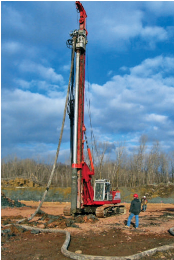
DGI-Menard installed Controlled Modulus Columns to improve the ground at a site with very soft fill.
