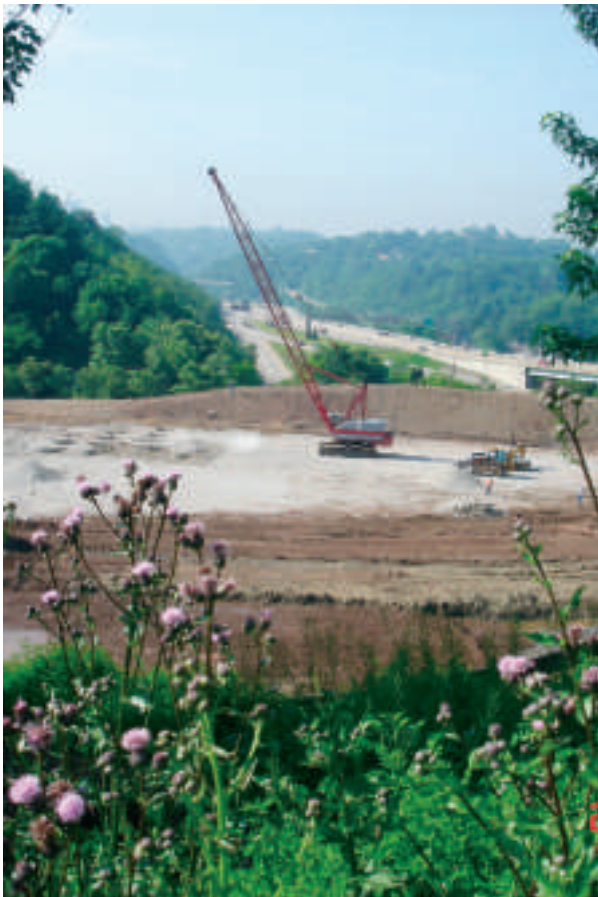
Compaction of the fill material across the building footprint was achieved using a 15-ton weight dropped from 70 feet.
