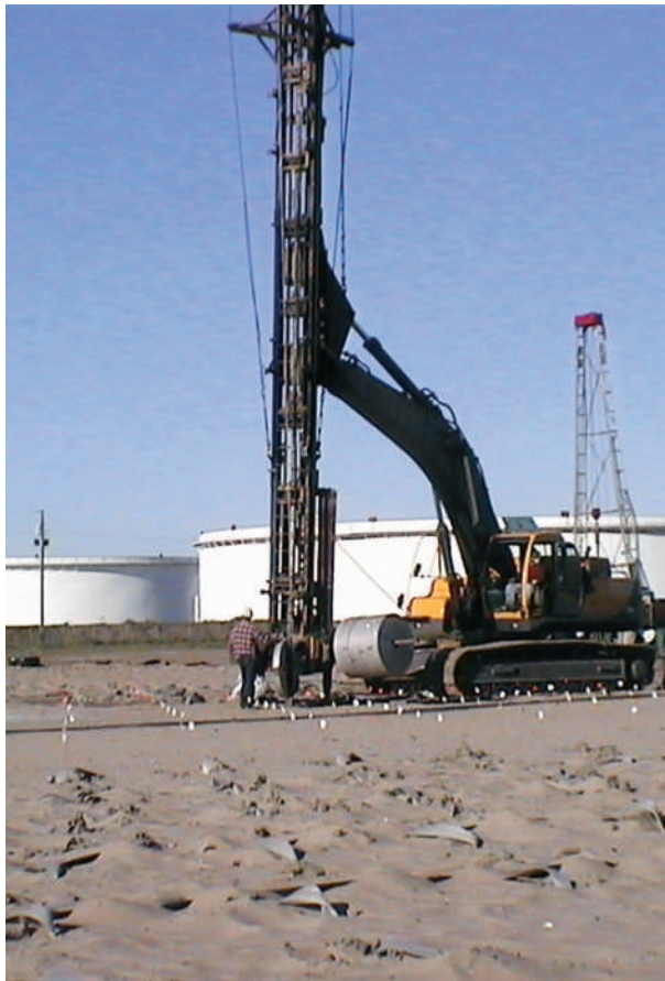
Installing wick drains to prepare the ground for the addition of several above ground storage tanks.
