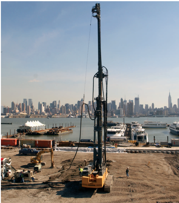
View of Menard's CMC operation showing grout delivery, pumping and drilling — directly across the Hudson River from midtown Manhattan.
