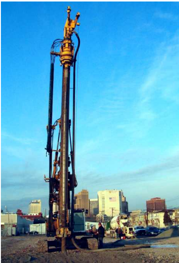
Menard installed over 750 CMCs to keep total and differential settlement to within project tolerances.
